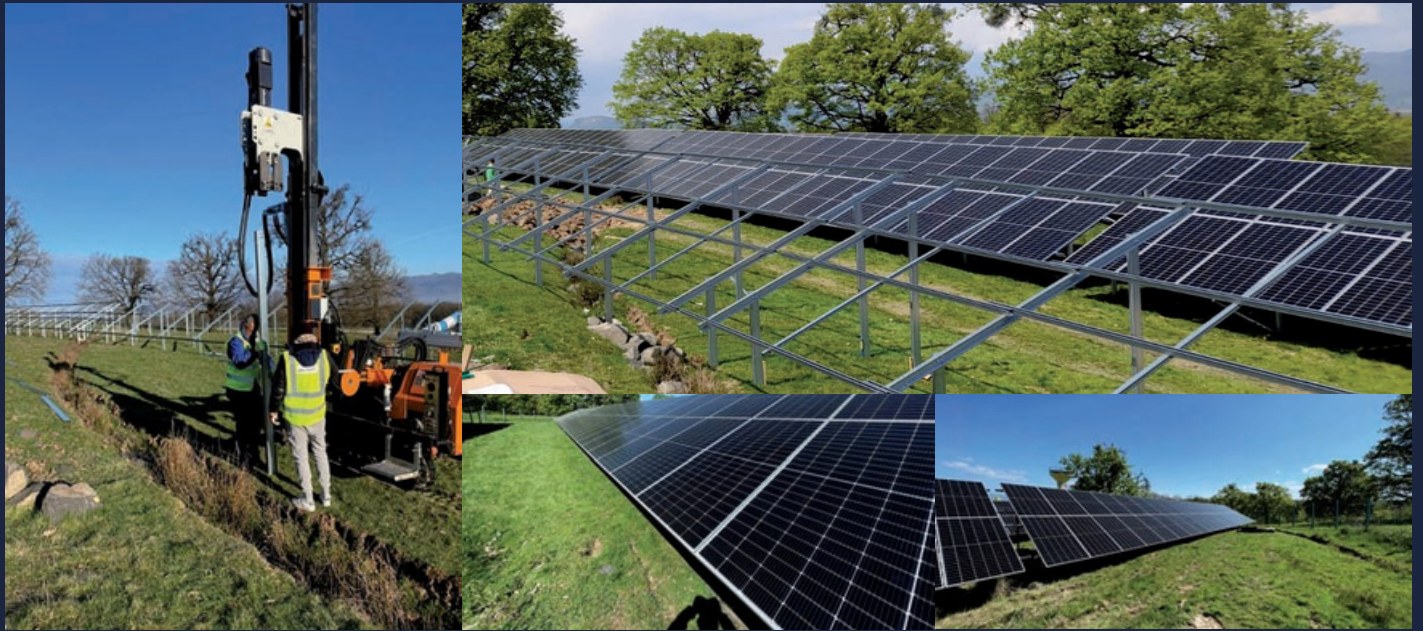
TIMCO SRL_ARSENAL PARC ORASTIE 517,75kWh
